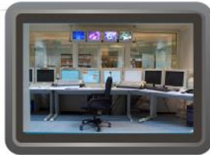
Central Control Room
